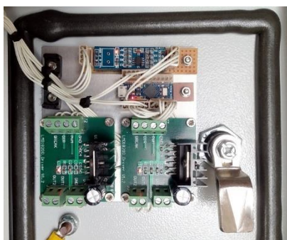
Figure 5 - Electronics package inside door
